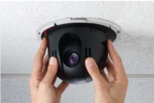
Put in the new "hot swap" PTZ camera module...
